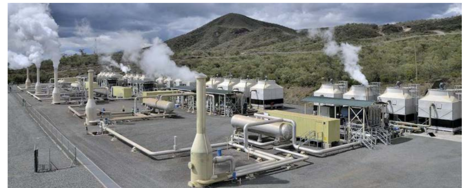
Well Head Geothermal plant in Olkaria.
