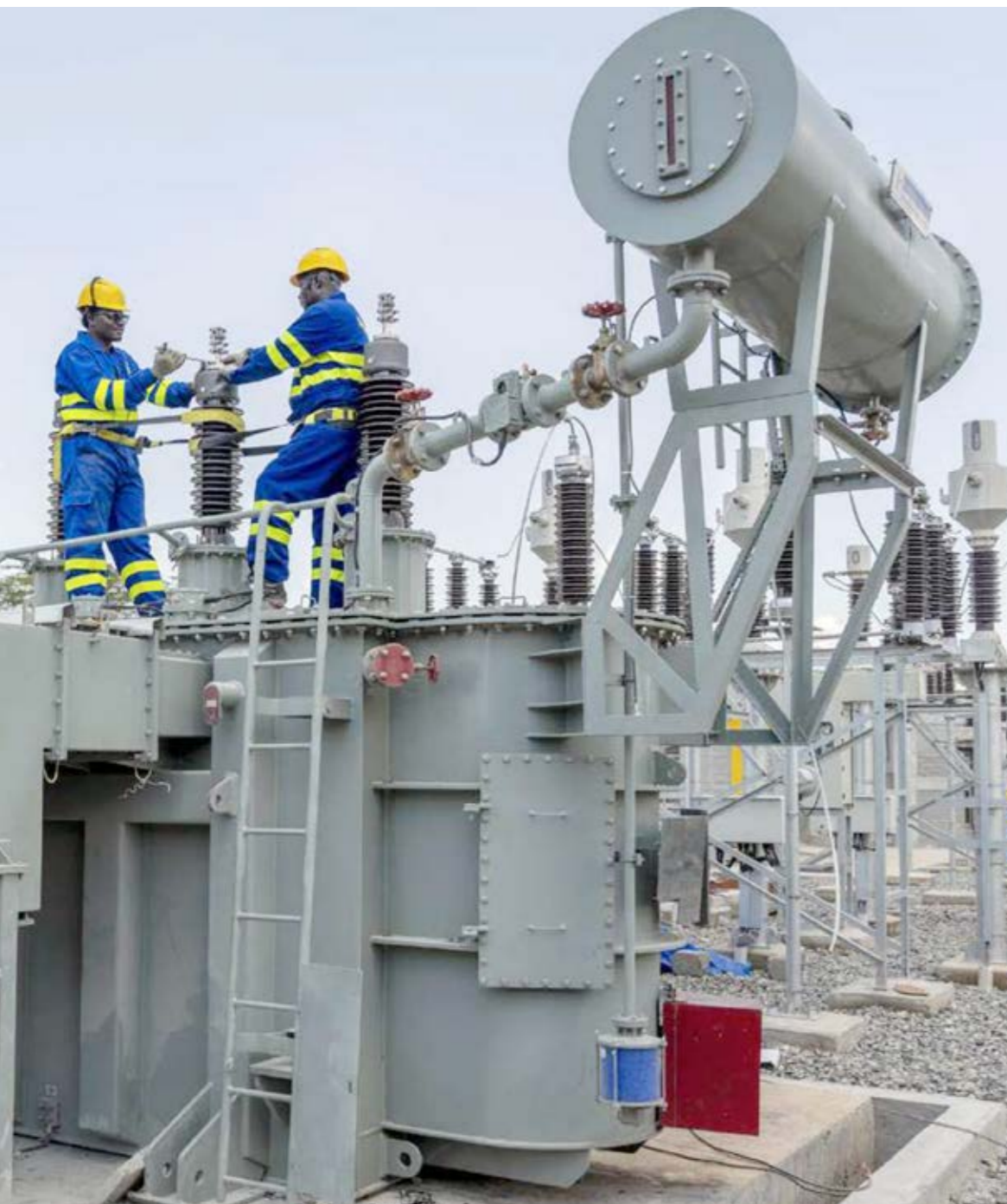
Power the nation: The central construction team implements strategic infrastructural projects to strengthen and expand the grid.
