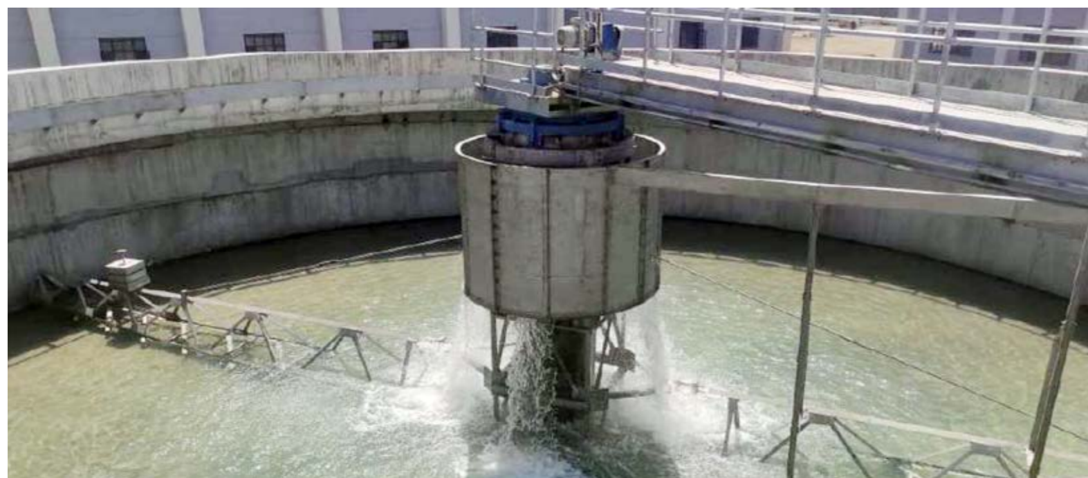
Waste not: A Common Effluent Treatment Plant at Kinanie Leather Industrial Park in Machakos County.
