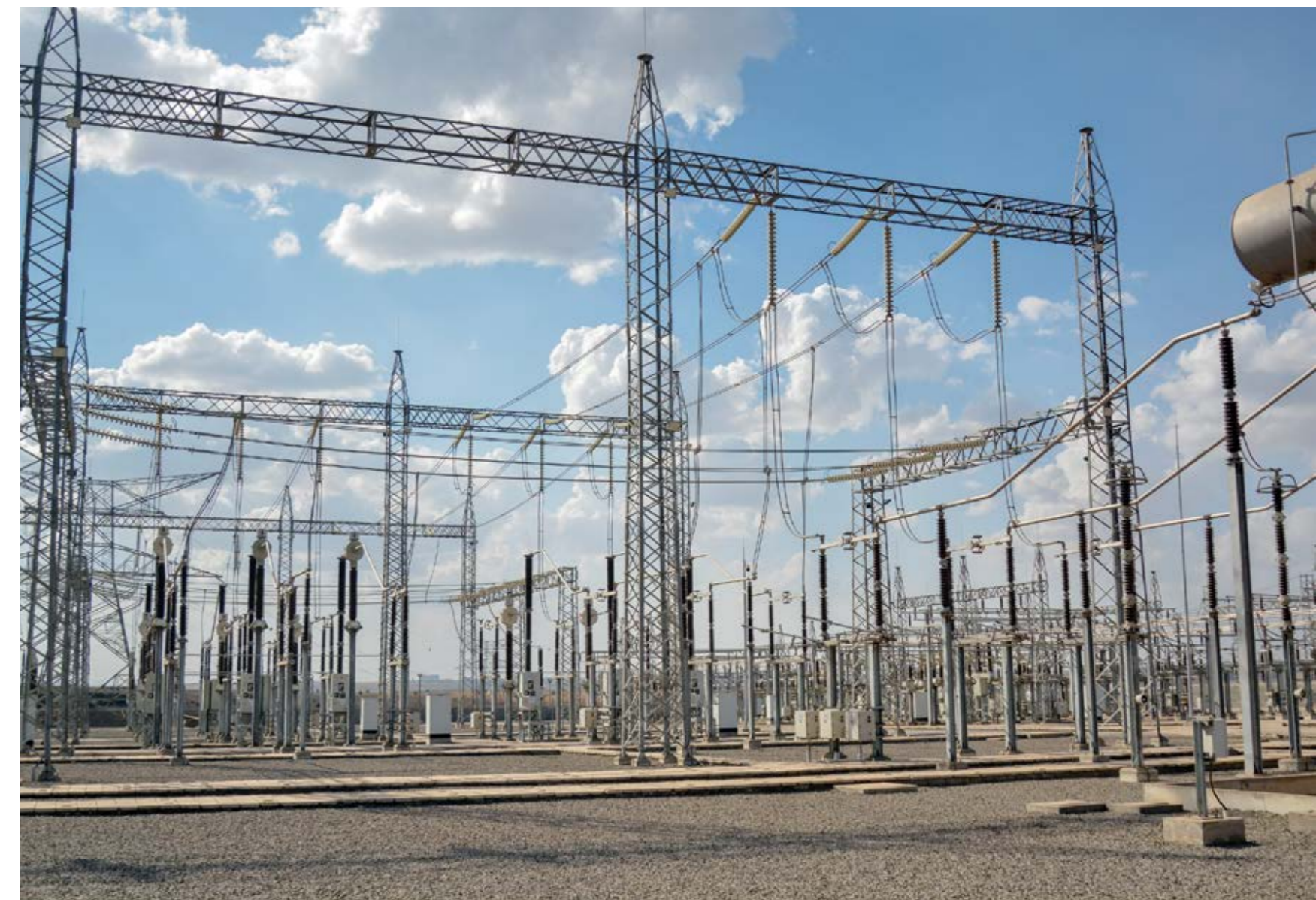
The Athi River Substation.
