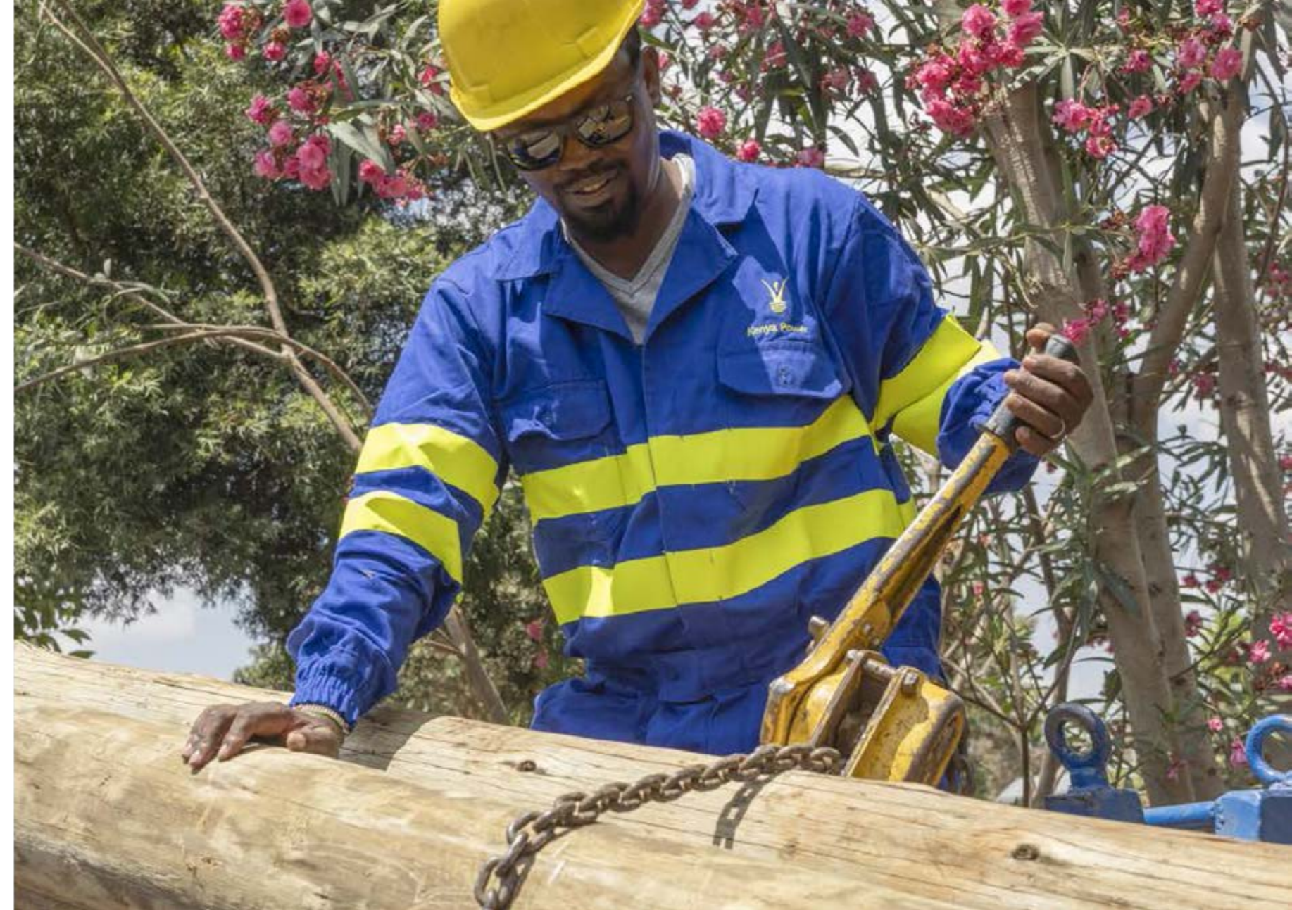
Power and light: They ensure power is supplied to light homes, schools and institutions and to run industries.
